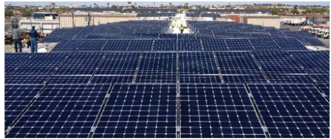
The City of El Paso partnered with Johnson Controls to install three solar arrays totaled 200 kW.
